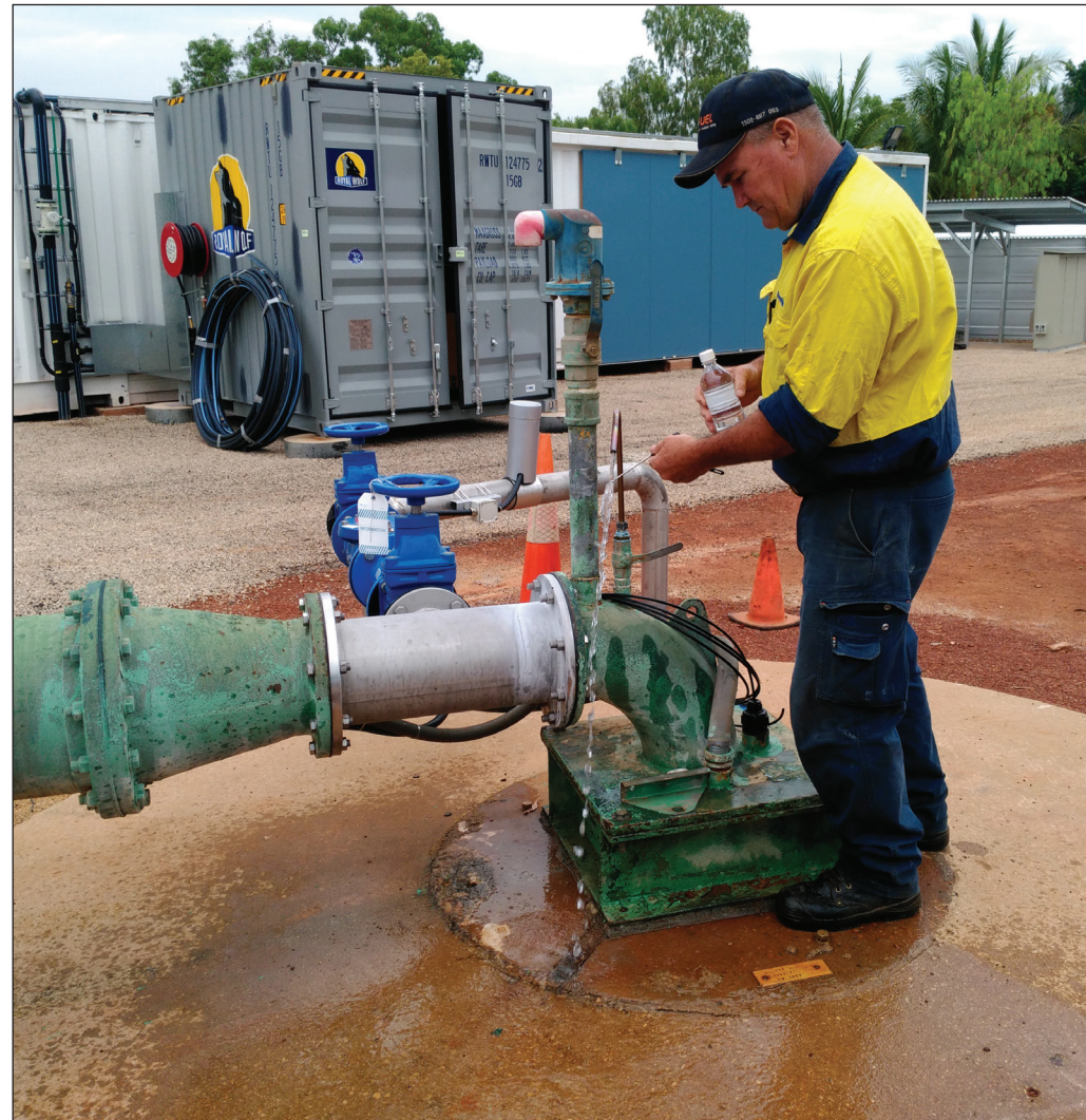
Water treatment plant operator Steve Murphy takes a sample of the treated water for testing.
